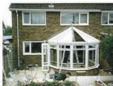
Note the stepped lead finishing detail at the rear of this conservatory where it adjoins the existing house wall
