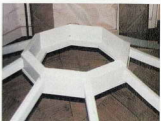
The dry fitting of a conservatory's lantern roof light in preparation for the installation of glazing panels
