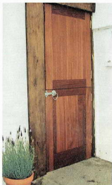
The finished door will need a weatherboard at the bottom, plus a smaller version on the top leaf
