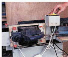
Planer and belt sander are easy to fit. Access to the NVR switch is good
